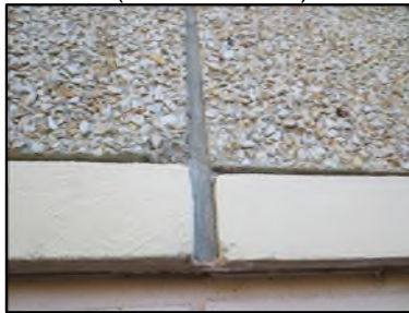
Photo N° 360 ECH-N°2 FACADE Murs Joint dilatation
