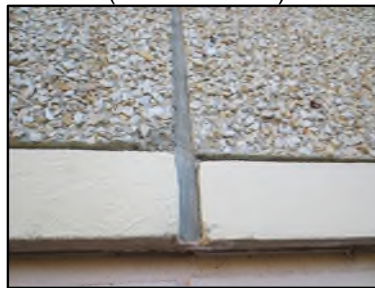
Photo N° 360 ECH-N°2 FACADE Murs Joint dilatation
