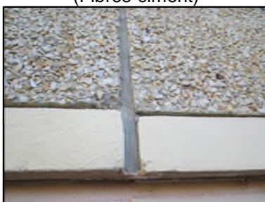
Photo N° 360 ECH-N°2 FACADE Murs Joint dilatation
