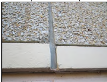
Photo N° 360 ECH-N°2 FACADE Murs Joint dilatation
