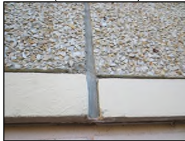
Photo N° 360 ECH-N°2 FACADE Murs Joint dilatation
