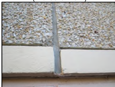
Photo N° 360 ECH-N°2 FACADE Murs Joint dilatation
