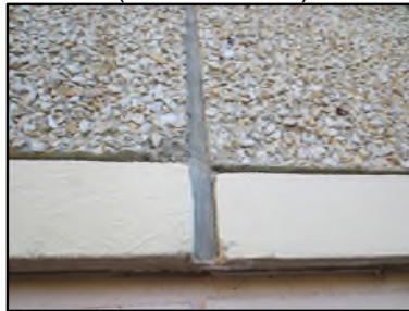
Photo N° 360 ECH-N°2 FACADE Murs Joint dilatation
