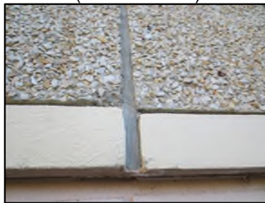
Photo N° 360 ECH-N°2 FACADE Murs Joint dilatation
