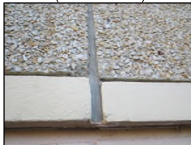
Photo N° 360 ECH-N°2 FACADE Murs Joint dilatation
