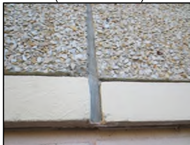
Photo N° 360 ECH-N°2 FACADE Murs Joint dilatation
