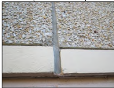
Photo N° 360 ECH-N°2 FACADE Murs Joint dilatation
