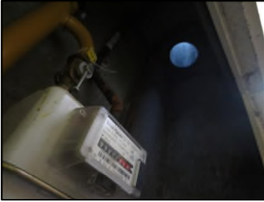
Photo N° 344 AMIANTE CIMENT -- Gaine Technique 4 Gaines & coffres verticaux Ventilation haute (Fibres- ciment)
