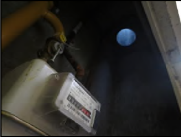
Photo N° 344 AMIANTE CIMENT -- Gaine Technique 4 Gaines & coffres verticaux Ventilation haute (Fibres- ciment)
