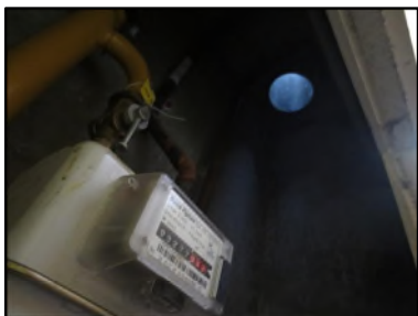
Photo N° 344 AMIANTE CIMENT -- Gaine Technique 4 Gains & coffres verticaux Ventilation haute (Fibres- ciment)
