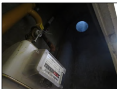
Photo N° 344 AMIANTE CIMENT -- Gaine Technique 4 Gains & coffres verticaux Ventilation haute (Fibres- ciment)
